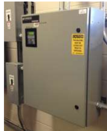
Figure 8 – Prime mover variable frequency drive
